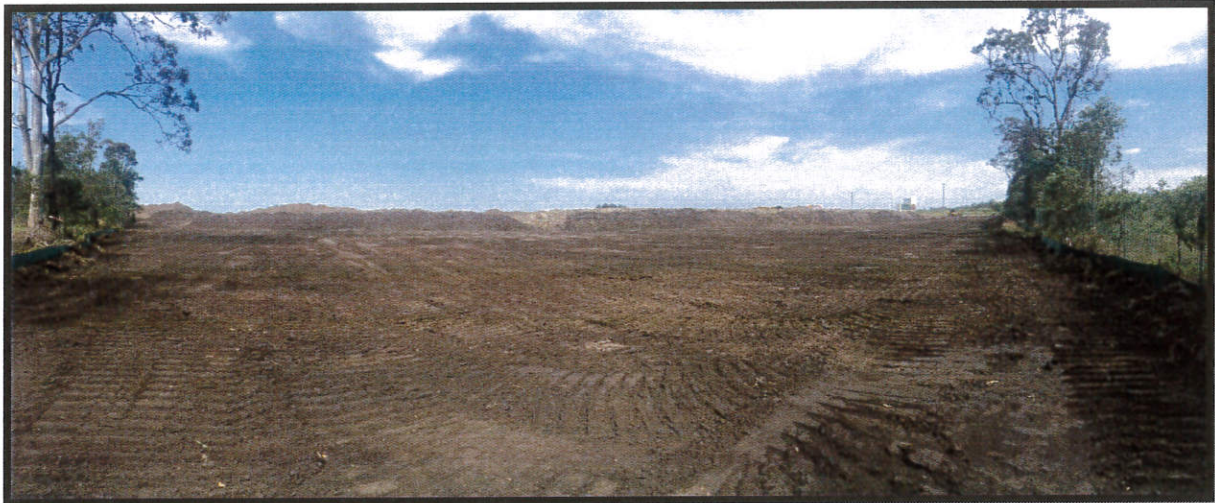
Picture 2: View of the Stripped Surface Prior to the Placement of Fill
