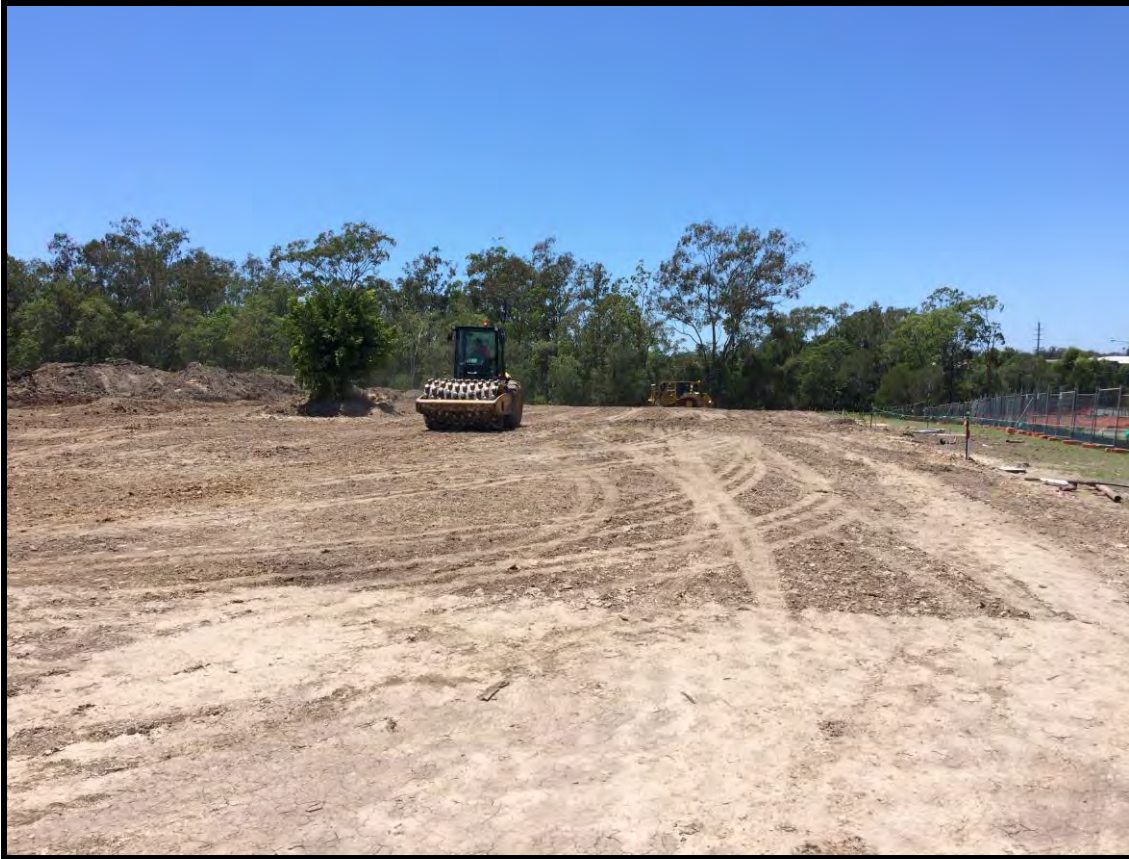
Picture 2: View of the Stripped Surface Prior to the Placement of Fill
